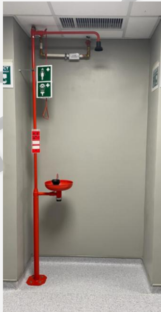
Safety shower at corridor
