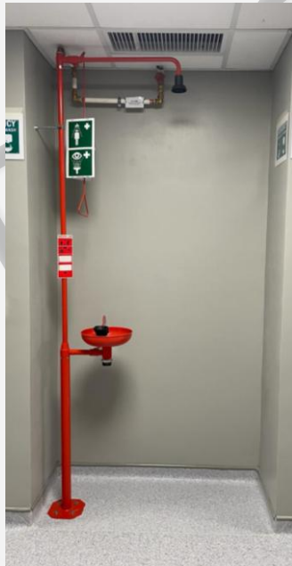
Safety shower at corridor
