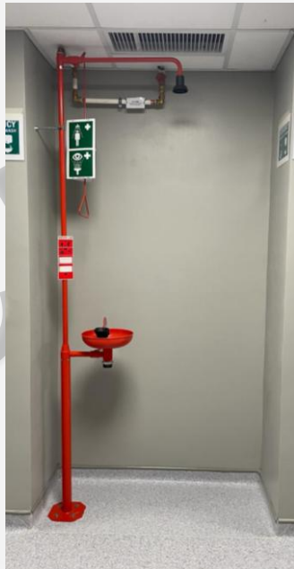
Safety shower at corridor
